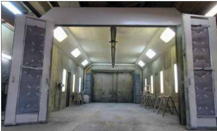
Drive-Through PAINT BOOTH
