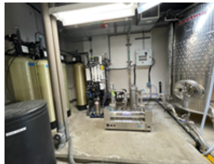
Reverse Osmosis System
